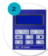
Eddy 5 control panel
